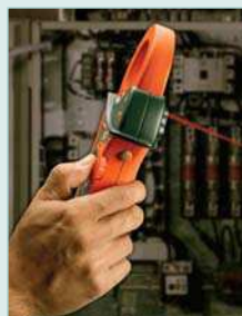
Built-in IR Thermometer with laser pointer is an excellent troubleshooting tool for locating hot spots and overheating motors.
